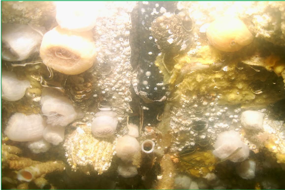
Figure 2-11. Marine growth near pontoon joint on Hood Canal Bridge, Washington (adapted from Anchor 2008).
